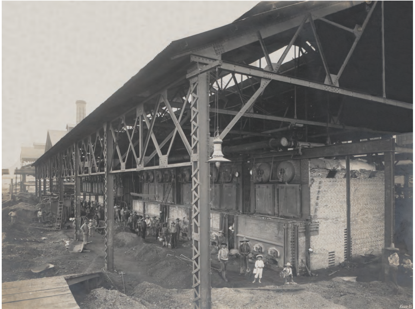
Fundidora Monterrey [spelled Monterey by Kahlo], "instalación de calderas" (year unknown)
